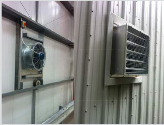
Liberator powered ventilator at Liverpool Parcelforce
