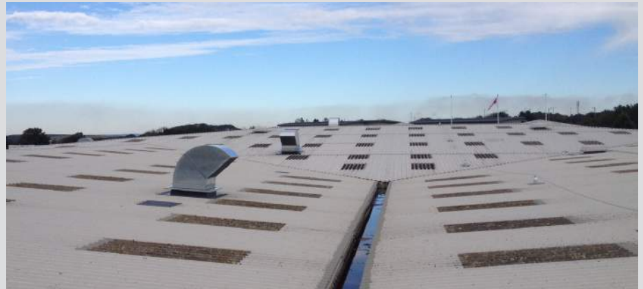
Mechanical air inlet at Bodmin Parcelforce
